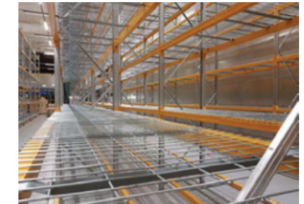
5 SHELVES Our sturdy shelves are made from steel mesh, which allows light as well as water from sprinklers to penetrate.
